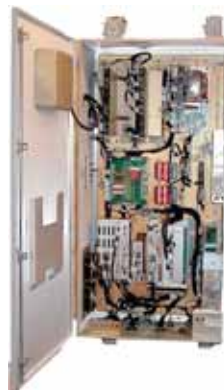
Pedestal Electronics Cabinet (PEC)
